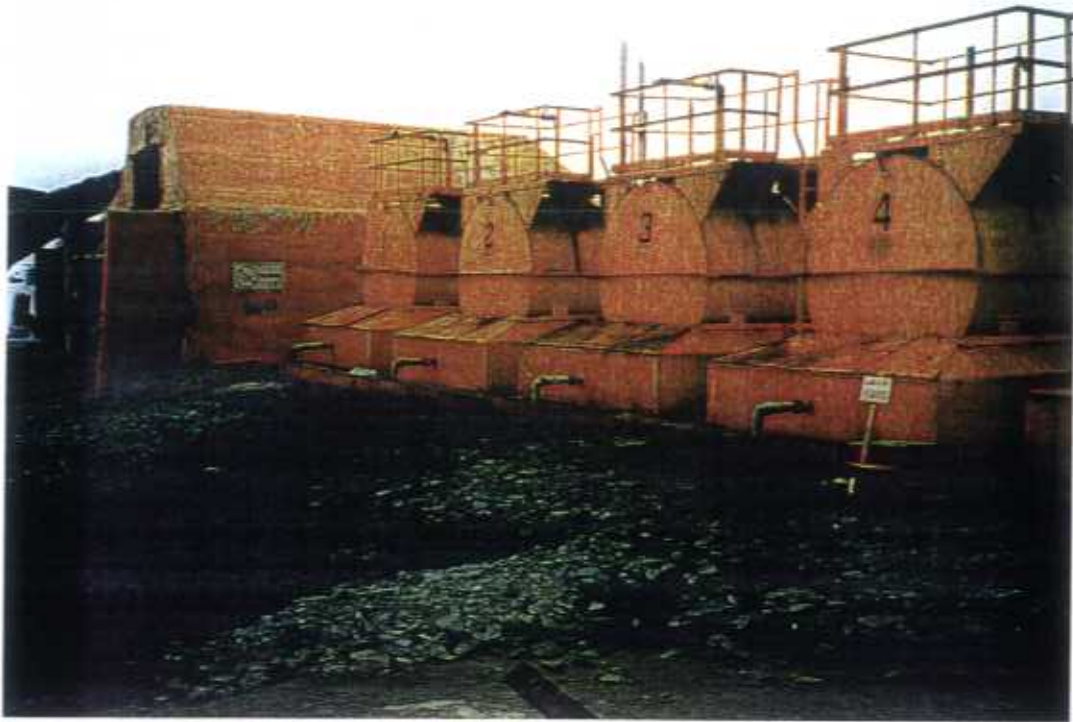
Bulk Fuel Tank with Bund Covers
