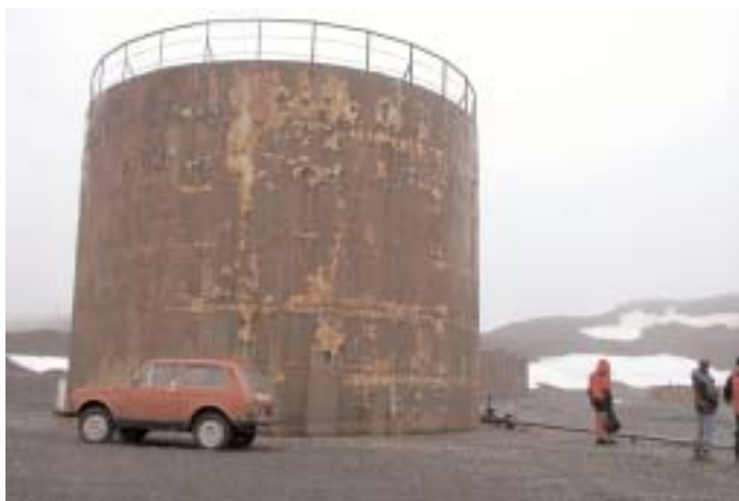
One of the large (250,000 litre) bulk fuel tanks at Rocky Cove, North of Bellingshausen.
