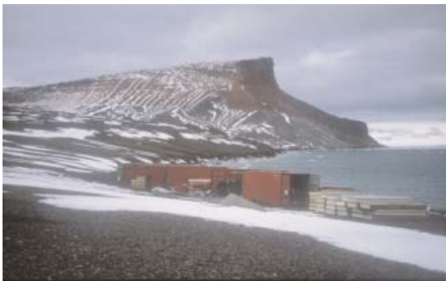
Containers offloaded on the beach for the construction of the new Czech Station on James Ross Island. Looking west towards Bibby Point.
